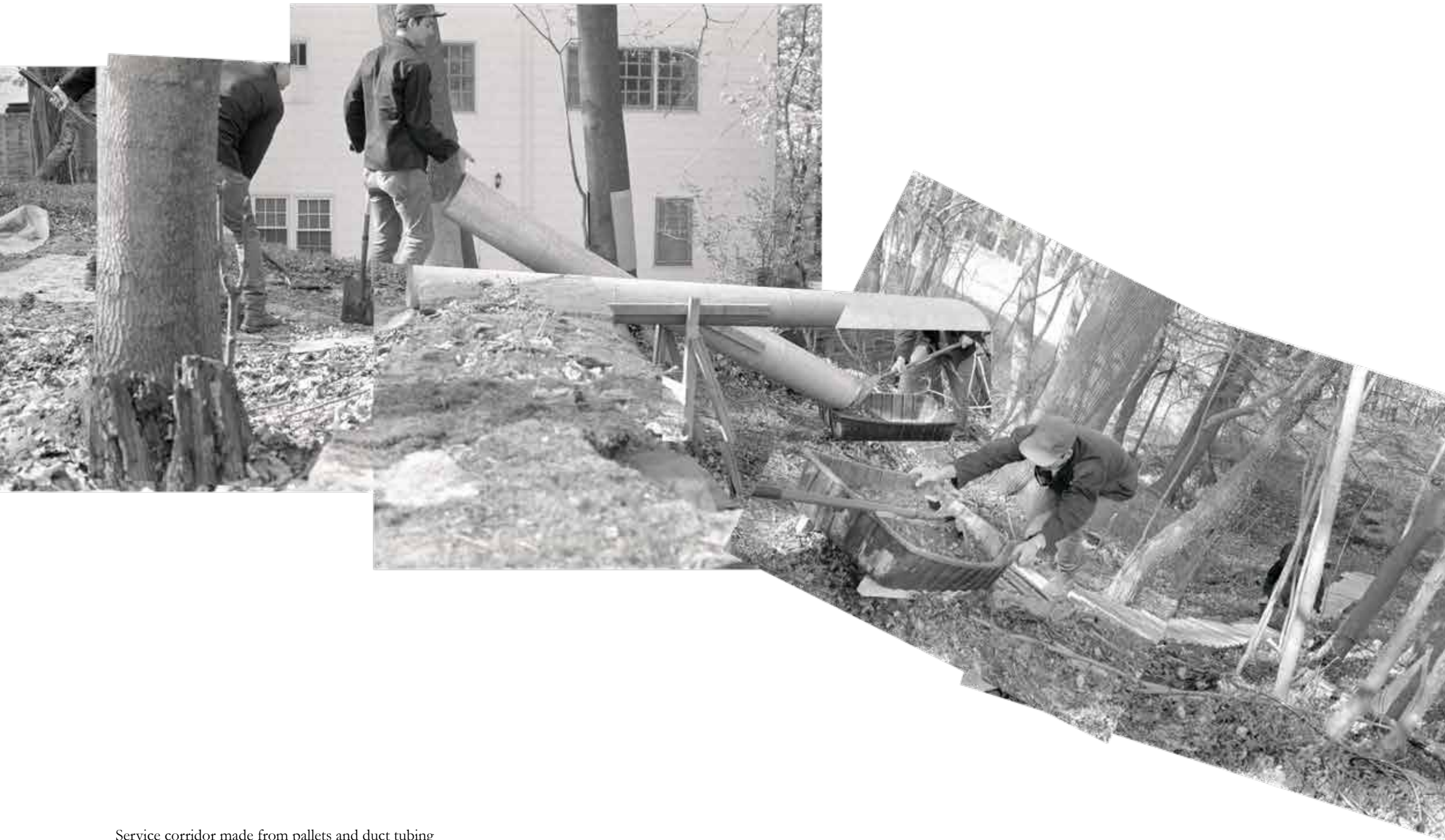
Service corridor made from pallets and duct tubing
